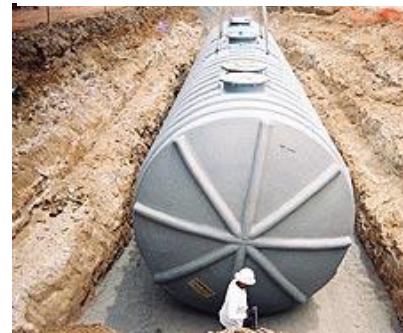
Figure 24 - Example Thermal Energy Storage Tank
