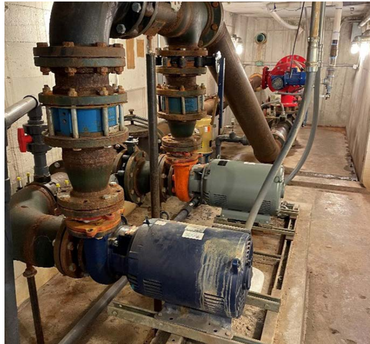
Pump station with filtration
